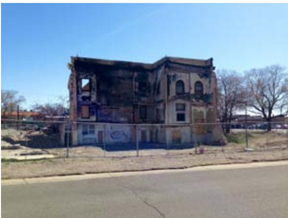
Image 3. White Hall as it stands today, with a demolished west-facing wall and open pit.
